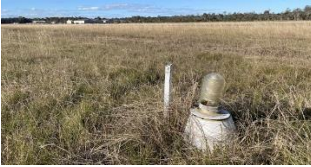
Figure 10 - Airport lighting (inoperable)
